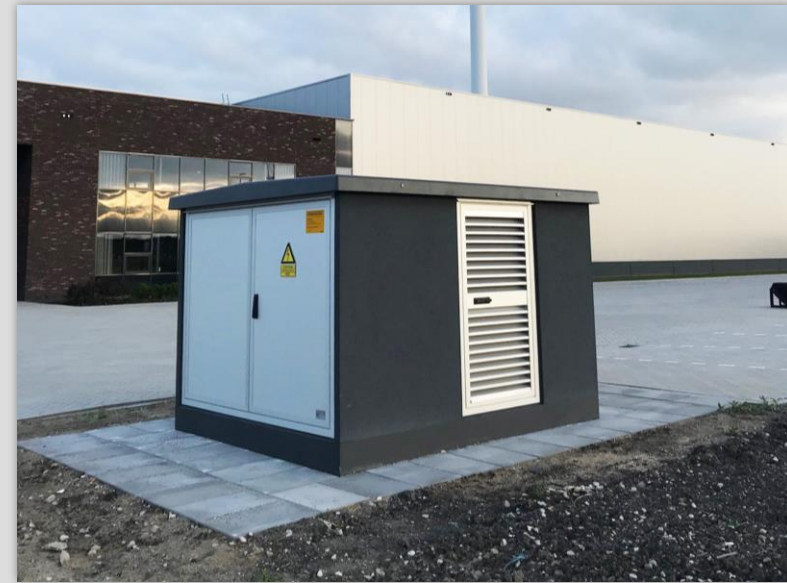
Elektrahuisje (MS-LS station)
